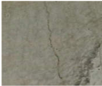
Figure 2. Cracked Concrete on the 27th Floor of The Newton 2 Apartment Project (analysis results)
