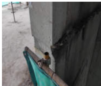
Figure 4. Concrete Deformation On The 20th Floor Of The Newton 2 Apartment Project (analysis results)
