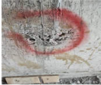
Figure 3. Concrete Honeycomb or Voids on the 19th Floor of The Newton 2 Apartment Project (analysis results)
