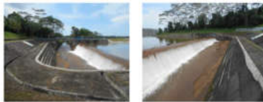
Figure 6 Dam Spillway Conditions
