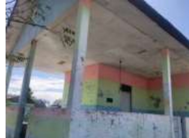
Figure 2. Posyandu building built through PNPB Mandiri Rural FY 2011
