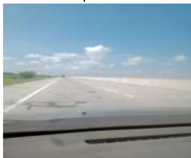
Figure 2. Uneven Toll Road Conditions
