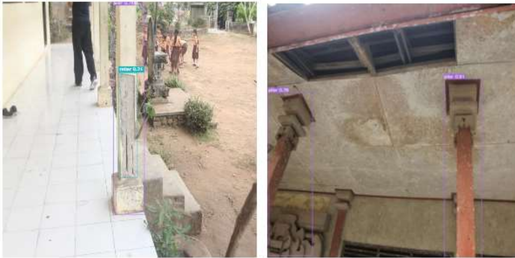
Figure 6. Detection Result for Pillar and Rebar Defects
