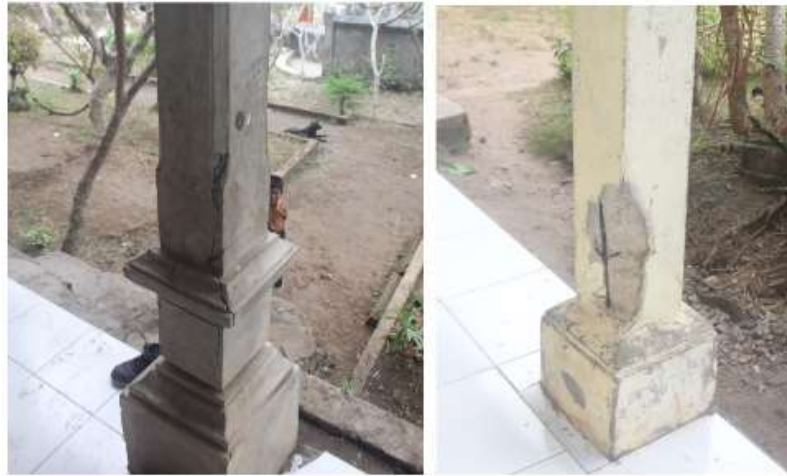
Figure 2. Samples of Pillars Photos and its defect
