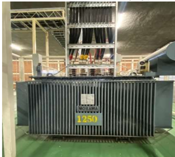
Figure 1. 1250 KVA Transformer at PT USDF
