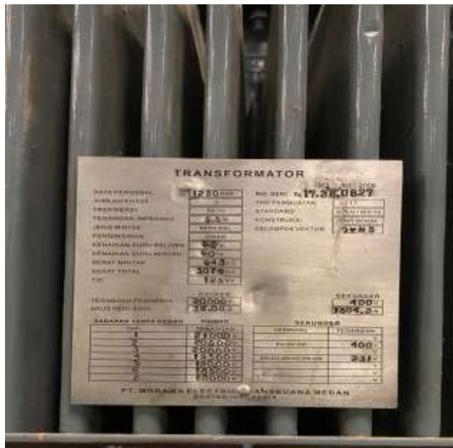
Source: Researcher Documentation (2025) Figure 2. Name Plate 1250 KVA Transformer at PT. USDF
