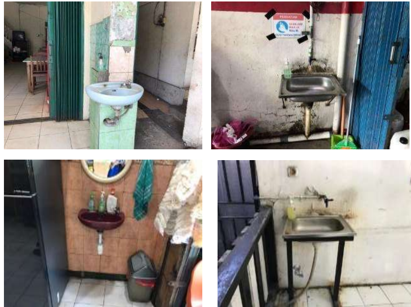
Figure 2 Hand washing facilities in each restaurant
