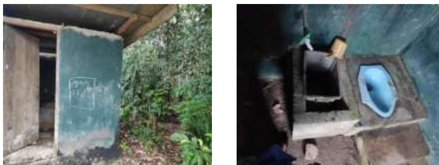
Figure 3 Existing facilities in the school toilet
